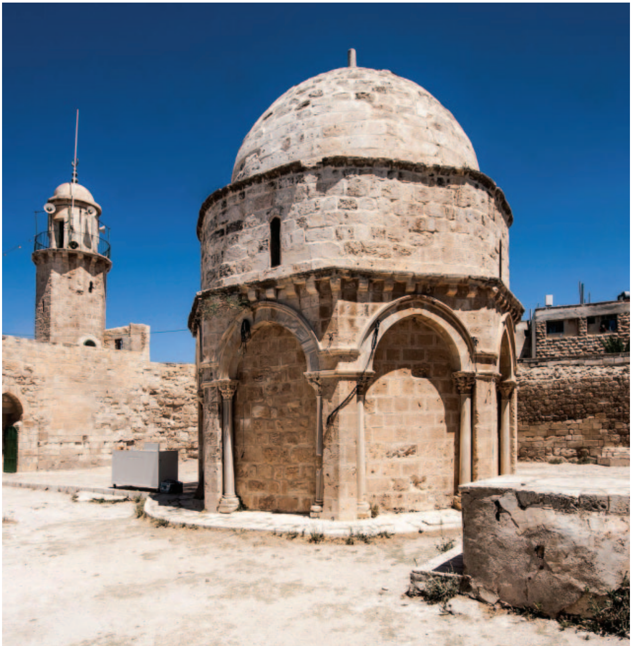
The Chapel of the Ascension on the Mount of Olives renovated by the Hashemite Restoration team of the Jerusalem Awqaf 2015–2017.
